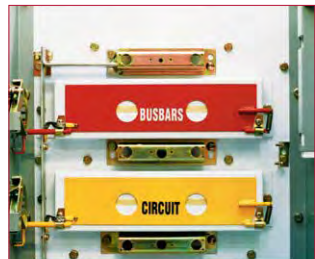
Circuit breaker compartment showing the orifice safety shutters and associated operating mechanism.
